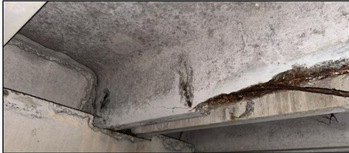
Figure 5-9: Bridge No. 070018 end region deterioration
