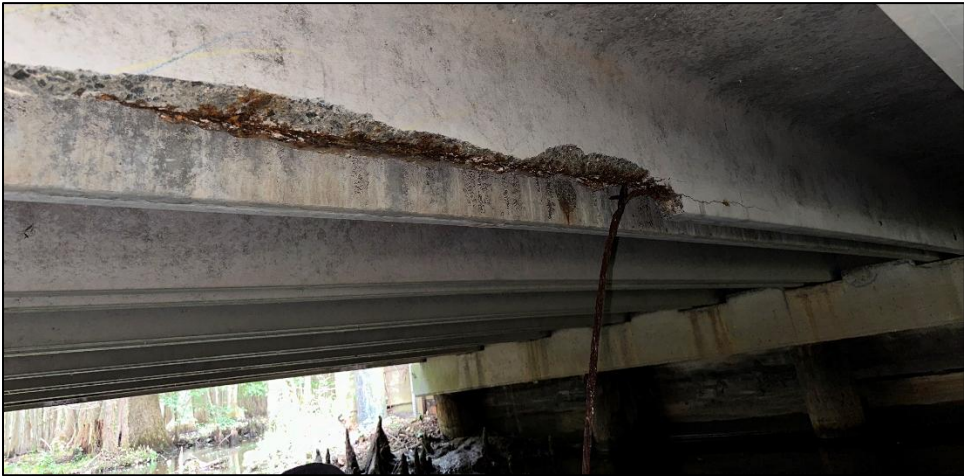
Figure 1-1: Example of a deteriorated prestressed concrete C-channel bridge beam (Bridge No. 070018)
