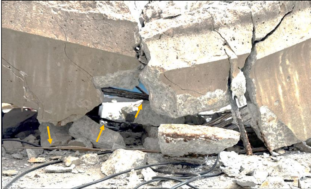
Figure 5-3: WCS1 internal prestressing strand corrosion
