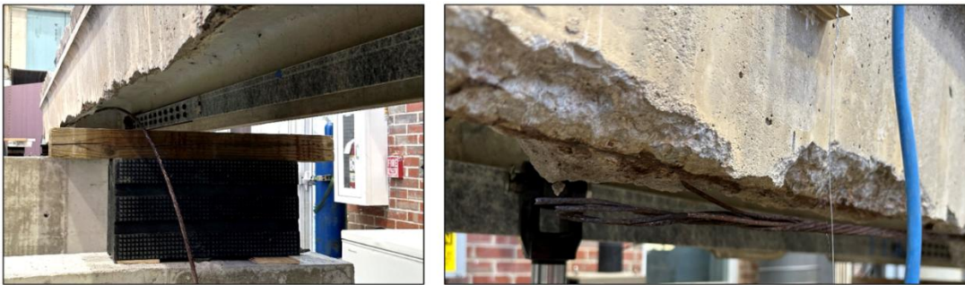
Figure 4-10: WCS2 bottom right prestressing strand rupture
