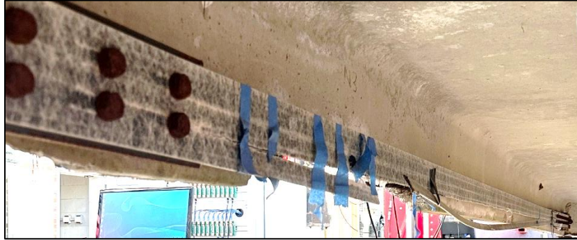
Figure 5-1: FRP plate damage prior to testing in SCS2
