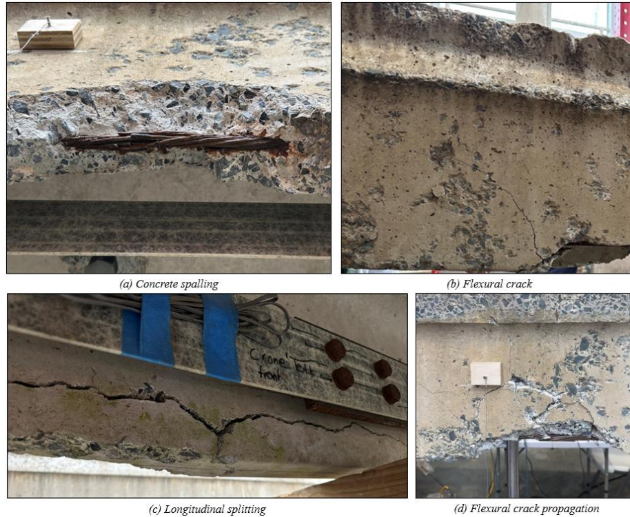
Figure 5-7: Damage signifying nonlinearity in a strengthened channel beam
