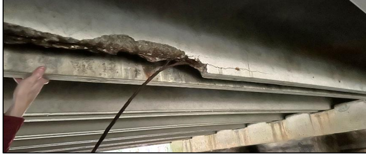
Figure 5-8: Bridge No. 070018 with a ruptured prestressing strand
